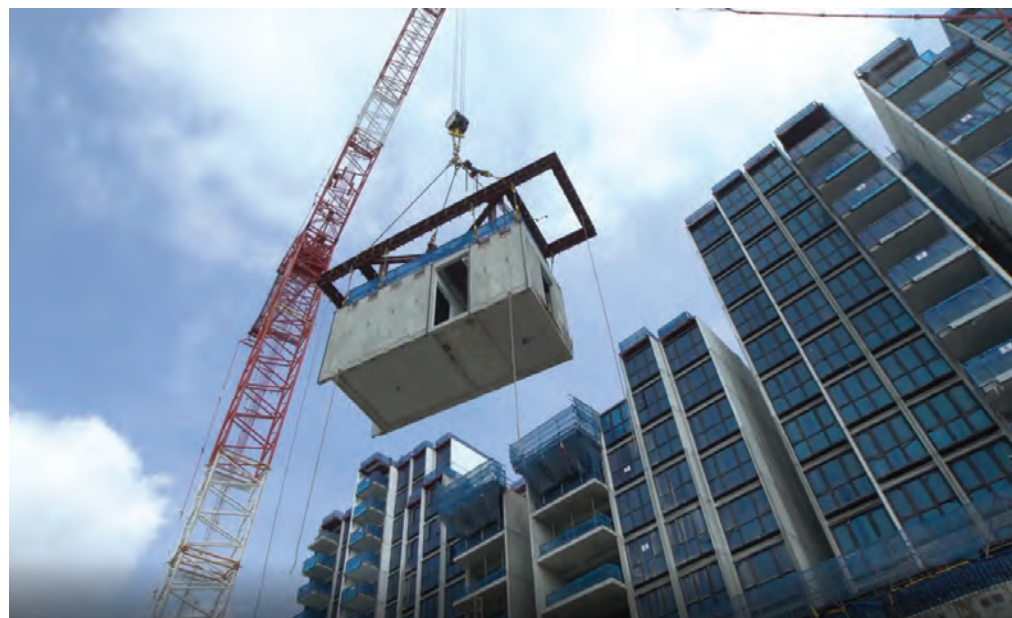
KaTRIS has developed a suite of solutions with its industry partners to improve productivity in PPVC installation. This construction method is increasingly popular in Singapore.
