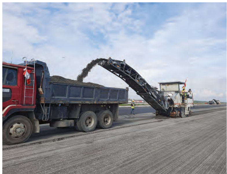
TOP AND ABOVE: The rehabilitation of runway 1 at Kuala Lumpur International Airport involved a total of 44,000 cu m of asphalt to be removed and repaved. A fleet of machines from the Wirtgen Group worked on this project, including Wirtgen cold milling machines, Vögele pavers and Hamm rollers.
