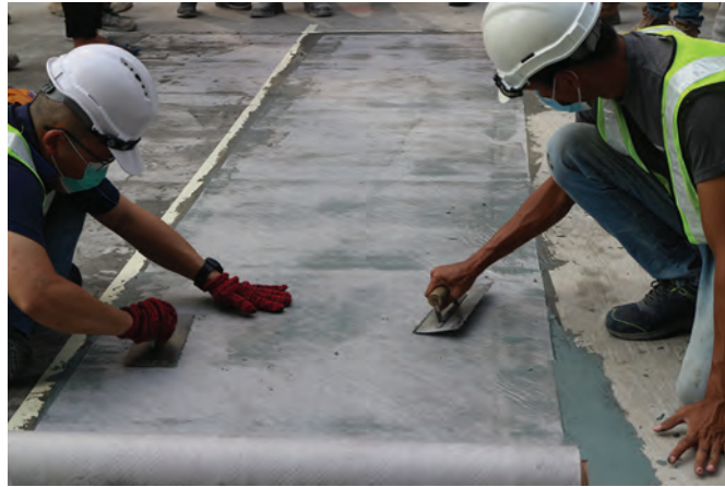
LEFT AND BELOW: The driveway was waterproofed with Mapelastick Smart cementitious mortar and Mapetex Sel polypropylene fabric.
