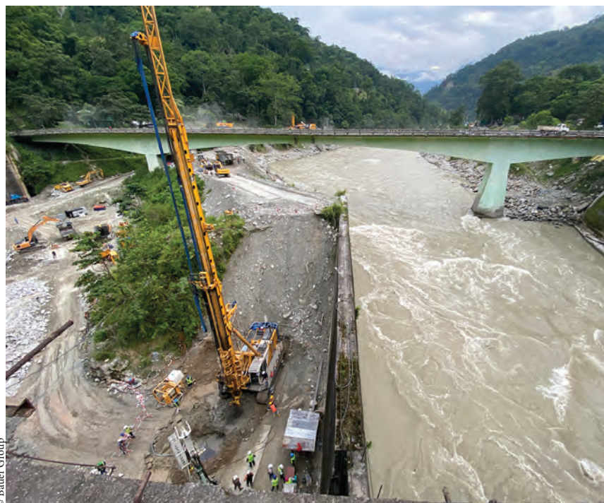
Bauer is undertaking the specialist foundation engineering and geotechnical work for the Teesta VI Hydro Electric project in the Indian state of Sikkim.
